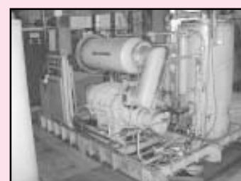
(3 Ea.) Dunham-Bush High Volume High Pressure Air Compressors, Model VAR-250LT2 with 250 H.P. Motors, Water Cooled, Compressor Models 2516DL63NOD. Design Pressure: 300 PSIG High Side, 250 PSIG Low Side
