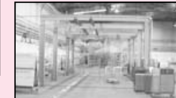
Overhead Rail System with Chain Falls and Electric Hoists To Do Engine Work
