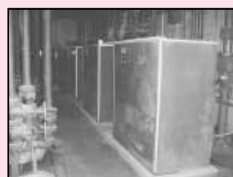
(3 Ea.) Zurn Model R360W Compressed Air Dryers MWP-200 PSIG Continuous Duty Capacity Inlet Air 100 Degree F, 1,250 SCFM @ 60 PSIG Corken Model DA390M9F BAB High Pressure Air Compressor, Water Cooled with 15 H.P. Motor
